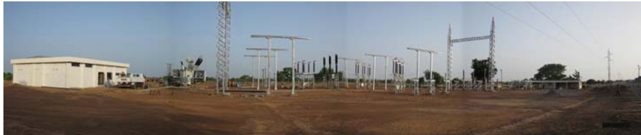
Newly installed Zebila sub-station in Ghana
